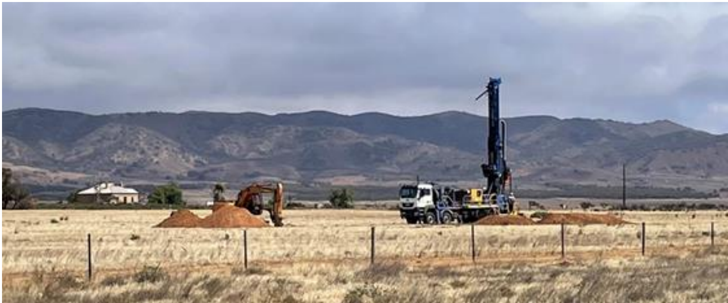
Photo: Drill rig on location at hole 1 (P01) of the Orroroo maiden drilling program.
